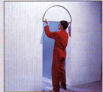
8. Arches: The shape of the opening is cut and a metal sheet inserted to act as a curved shutter.
