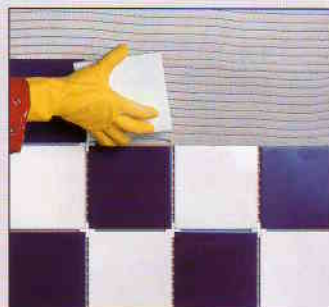
18. Interior tile fixing without prior plastering; applied directly to the isorast wall.
