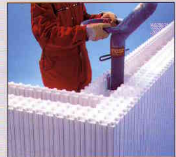
12. Concreting with the isorast nozzle and ready-mix concrete or dry concrete from the silo.
