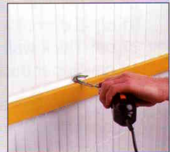
16. Forming service chases in minutes is possible with the isorast hot wire cutter.
