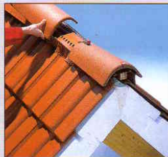
14. isorast roof insulation panels are nailed on to rafters and then tiles overlaid. U-values up to 0.1w/m 2 K are possible.
